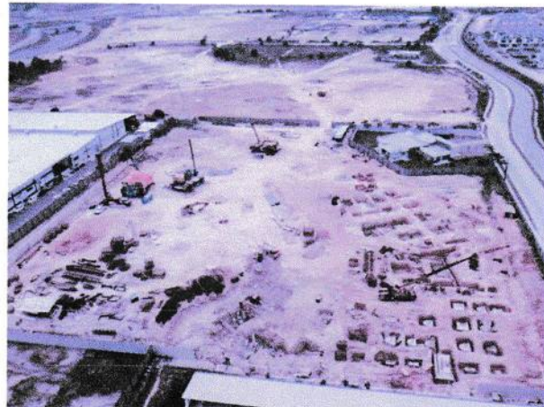
Jack-in Pile Design and Construction for High-rise Buildings - A Malaysian Consulting Engineer's Perspective, after C. M. Chow and Y.C. Tan (2021)
